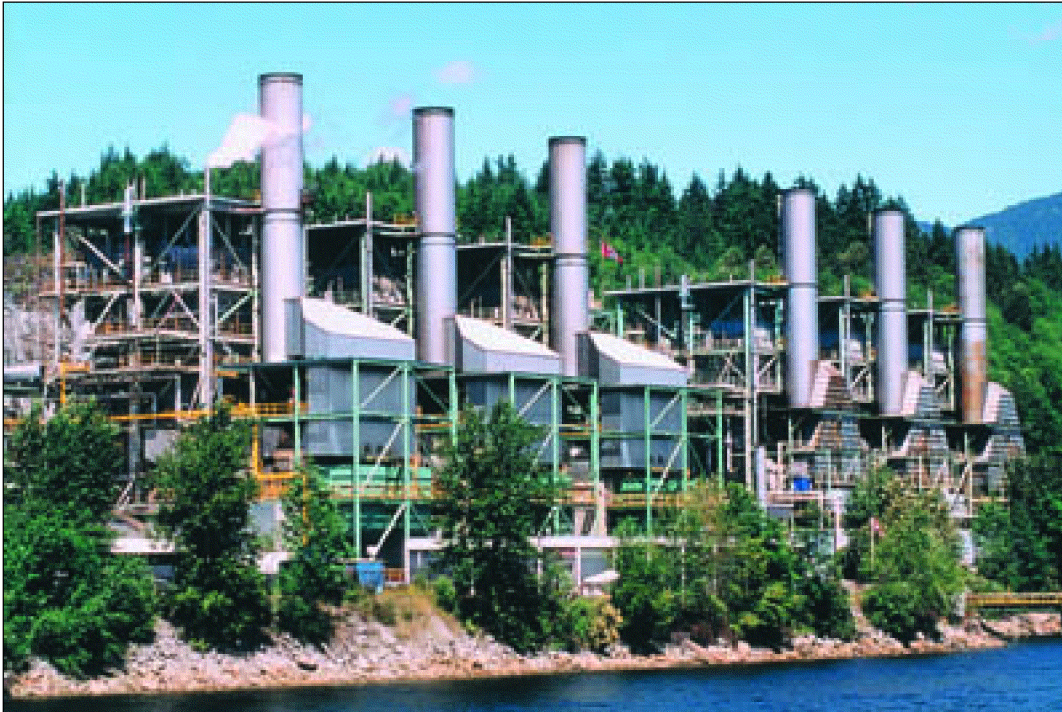
Three Selective Catalytic Reduction systems are installed at B.C. Hydro's Burrard Station, a natural gas-fired plant located near Vancouver.
