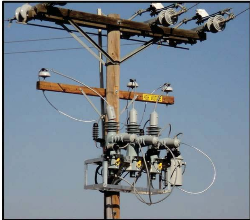
Recloser on Distribution Pole
