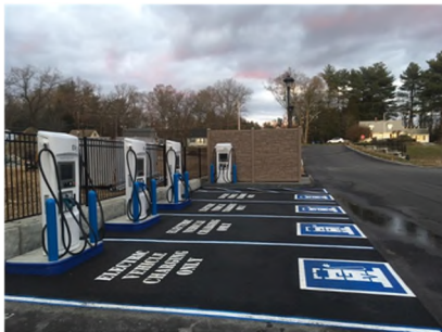
Electric vehicle charging station
