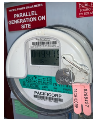
Smart meter for farm solar electric system
