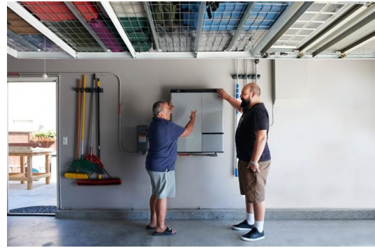
Customer discussing Brightbox solar battery system with neighbor in West Corona, California
