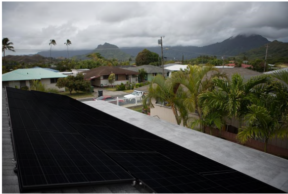
Solar installation in Hawaii
