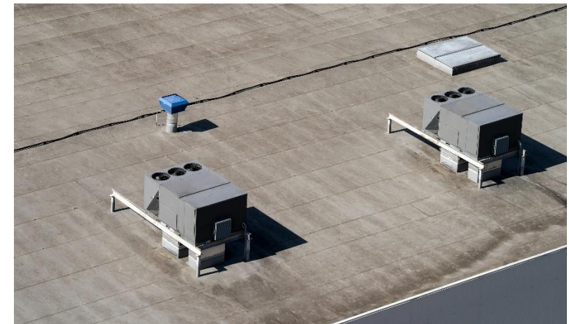
Image description: Example of rooftop units
