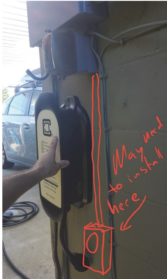
Figure 2: Max's EVSE Install Location
